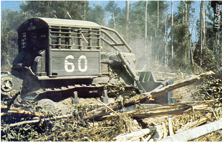
A modified D7E bulldozer equipped with a Rome Plow blade and an armored cab clears trees and brush. The vehicles became an effective tool for clearing roadside areas, hindering enemy ambushes, and limiting cover and concealment.
