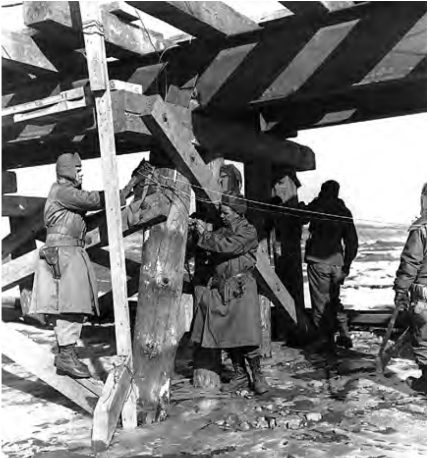
U.S. combat engineers place satchel charges on a railroad bridge near P'yongyang, preparing to destroy it to slow the Communist advance. (DA photograph)
