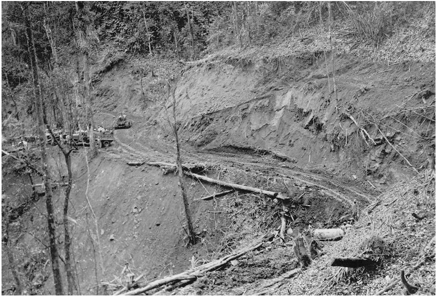
Army bulldozers constructing the Ledo Road cut a path through a hillside in the Indian jungle. (DA photograph)
